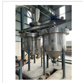
Caustic Wash Tank
