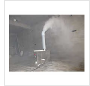
Cold Storage Humidifier Machine
