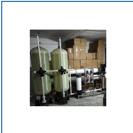
INDUSTRIAL 100 LPH RO PLANT
