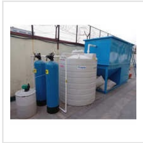
20 KLD Packaged Sewage Treatment
