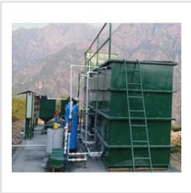
50 KLD Automatic Sewage Treatment
