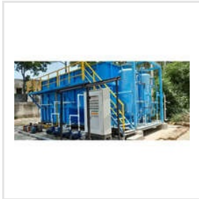
Commercial Sewage Treatment Plant
