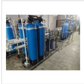
1000 LPH RO Plant
