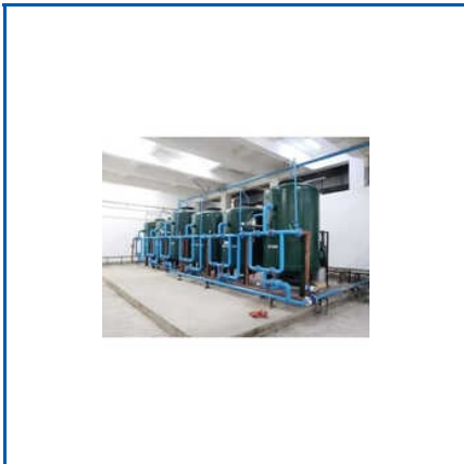
FULLY AUTOMATIC WATER TREATMENT PLANT
