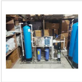
Commercial 250 LPH RO Plant
