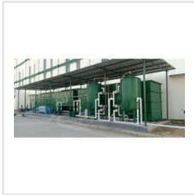
500 KLD Sewage Treatment Plant
