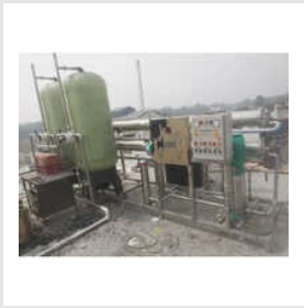
Commercial 5000 LPH Water Treatment Plant
