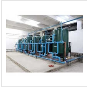
Semi-Automatic Water Softener Plant
