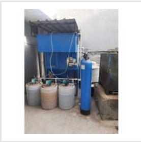
10 KLD Effluent Water Treatment Plant
