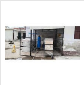
220V Water Treatment Plant
