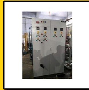
ELECTRICITY DISTRIBUTION PANELS
