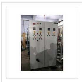
Electricity Distribution Panels
