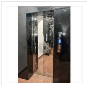
Office Passenger Elevator
