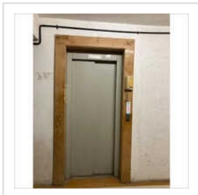
Hydraulic Home Elevator
