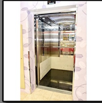
SHOPPING MALL PASSENGER ELEVATOR
