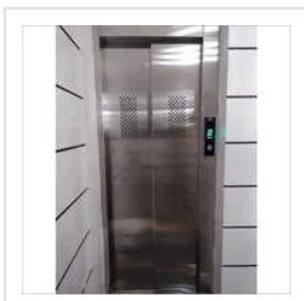
Office Stainless Steel Passenger Elevator
