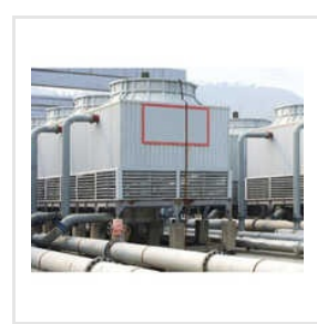
Industrial Cooling Tower
