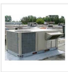
Roof Top Air Conditioner
