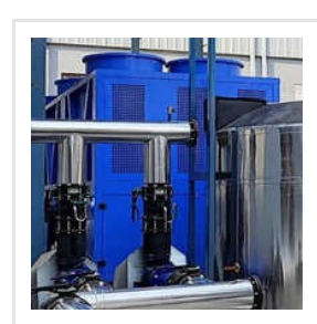
Industrial Process Cooling Chiller
