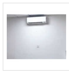
Split Air Conditioner
