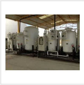
10 TPD CBG Commercial Project
