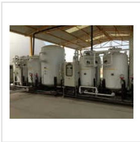
12000 M3 Natural Biogas Purification
