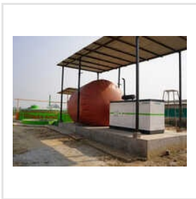
Commercial Bio Cng Plant
