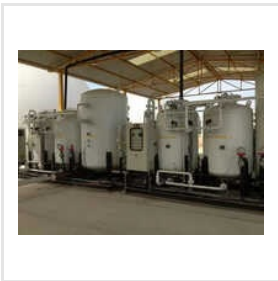
Biogas Power Generation Plant
