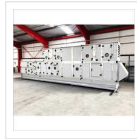
Air Handling Units
