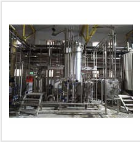
Brew Filtration Plant
