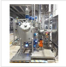
Cellar Ratio Controlled Dosing System
