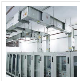
Busbar Trunking System
