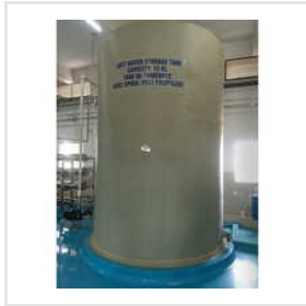
Soft Water Storage Tank
