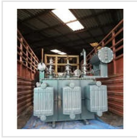
250 KVA Distribution Transformer
