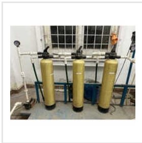
1000 LPH DM Water Plant
