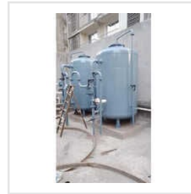
Effluent Wastewater Treatment Plant
