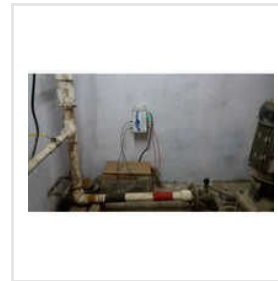
Electronic Water Softener Plant
