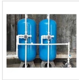
Swimming Pool Filtration Plant
