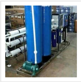
Industrial Water Treatment Plant
