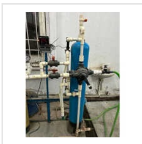
500 LPH Mix Bed Plant
