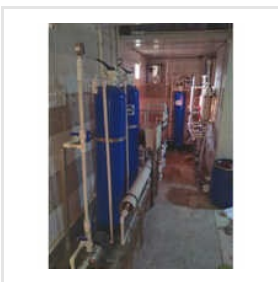
DM Water Plant
