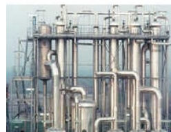
Industrial Zero Liquid Discharge Plant
