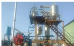
Evaporator With Thermic Fluid Heater
