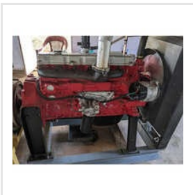
25 KVA Bio Gas Generator
