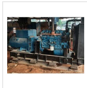
40 KVA Bio Gas Generator
