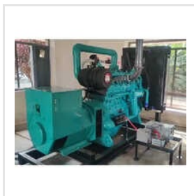
100 KVA Bio Gas Generator
