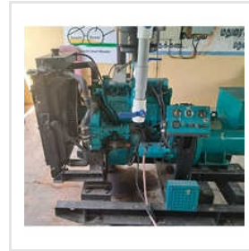
20 KVA Bio Gas Generator
