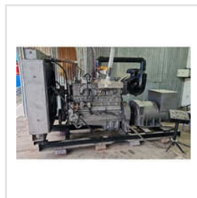
125 KVA Bio Gas Generator
