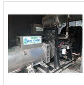
50 KVA Bio Gas Generator
