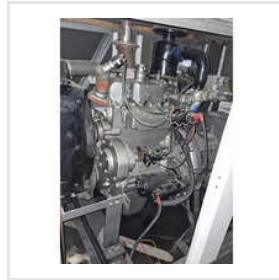
15 KVA Bio Gas Generator
