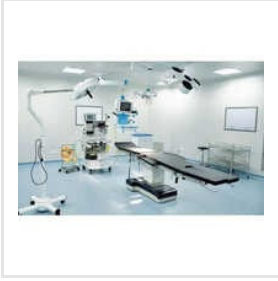
Modular Operation Theatre
