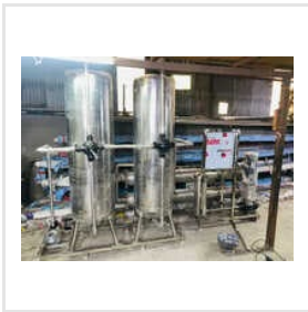
SS RO Plant
