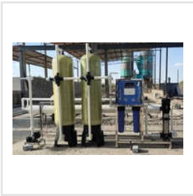
3000 LPH Industrial RO Plant
