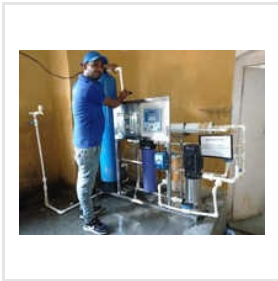
Industrial RO Plant Maintenance Service
