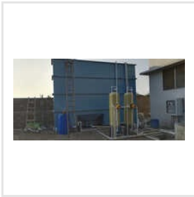
Packaged Sewage Treatment Plant
