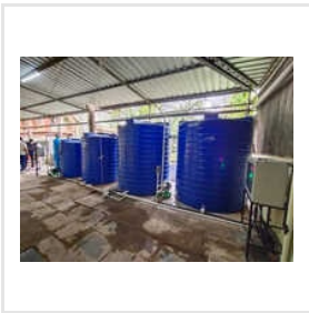
Water Waste Treatment Plant
