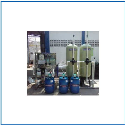
6000 LPH INDUSTRIAL RO PLANT
