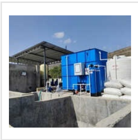
Industrial Waste Water Treatment Plant
