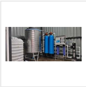
Commercial Ro Plant
