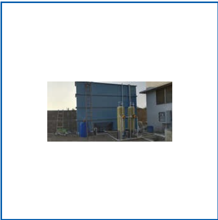
SEQUENTIAL BATCH REACTOR
