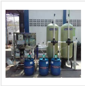
Industrial Ro Water Filter
