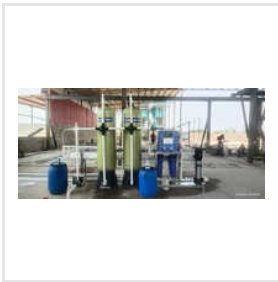
Industrial Ro Plant
