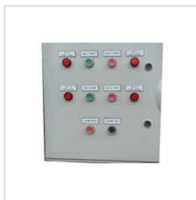
Silo Pneumatic Control Panel
