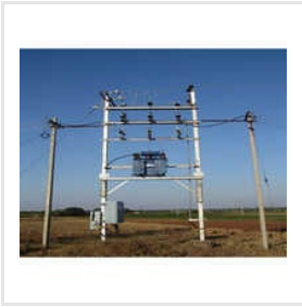
HT Line 11KV And 33KV Double Cast Iron
