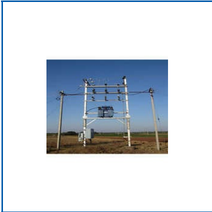
HT LINE 11KV AND 33KV DOUBLE CAST IRON ELECTRIC POLE
