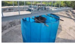
Central Drive Clarifiers
