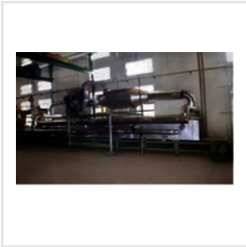
On Line Conveyor Oven
