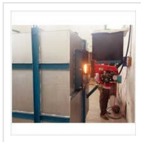
Electric Bell Furnace
