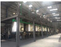
Sulphate Extraction Plant
