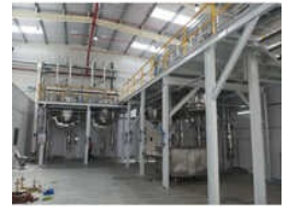
Vacuum Distillation Plant
