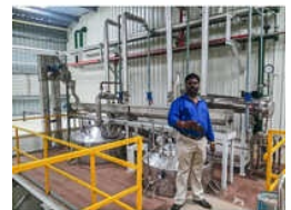
Spice Oil Distillation Plant
