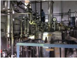
200 TPD Solvent Extraction Plant
