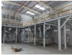
Essential Oil Distillation Plant
