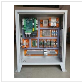
Parallel Wiring Elevator Control Cabinet
