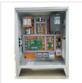
V3f Lift Control Panel
