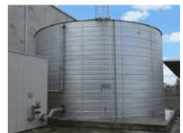
Industrial Zinc Aluminium Water
