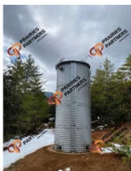
Zinc Aluminum Rain Water Storage Tank
