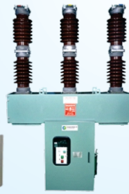
33KV / 11KV OUTDOOR VCB
