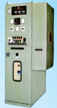
11KV VCB PANEL
