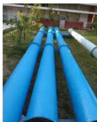
PP FRP Fume Exhaust Duct
