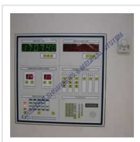
OT Control Panel
