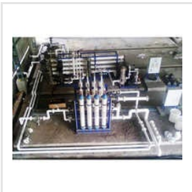
Condensate Polishing Unit
