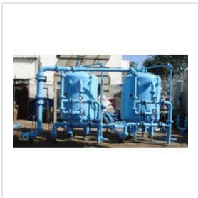
Pressure Sand Water Filter
