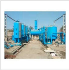
Electro Mechanical Equipment For Water
