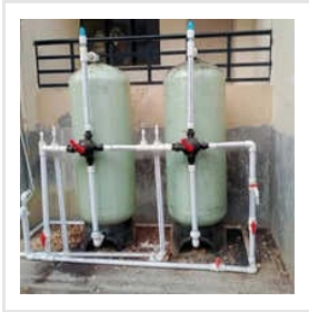
Iron Removal Filter Plant
