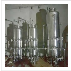
Water Softening Plant System
