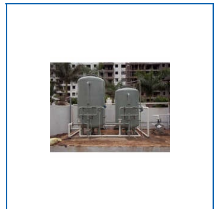
WATER RECYCLING SYSTEM
