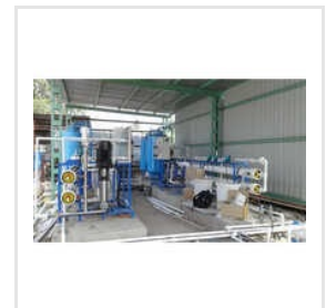
Automatic UF Plant
