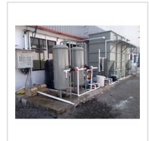
Package Sewage Treatment Plant
