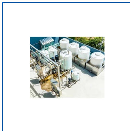
GRAY WATER TREATMENT PLANT
