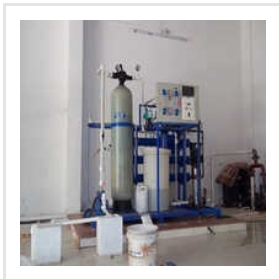
Reverse Osmosis Plants
