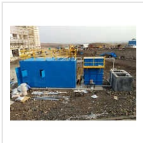
Containerized Sewage Treatment Plant
