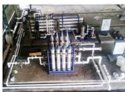
Condensate Polishing Unit
