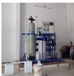
Reverse Osmosis Plants
