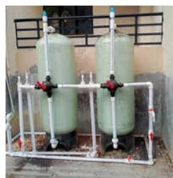
Iron Removal Filter Plant
