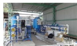
Automatic UF Plant
