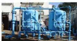
Pressure Sand Water Filter
