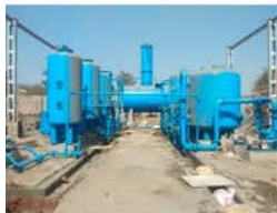
Electro Mechanical Equipment For Water
