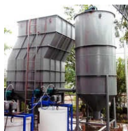
Lamella Clarifier System
