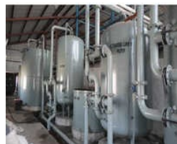
Water Softening Plant Installation
