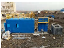
Containerized Sewage Treatment Plant
