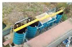
Waste Water Treatment Plant
