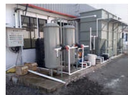
Package Sewage Treatment Plant
