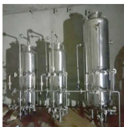
Water Softening Plant System
