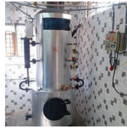
Wood Fired Steam Boiler
