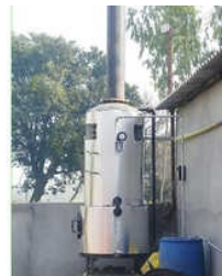
Industrial Non IBR Steam Boiler
