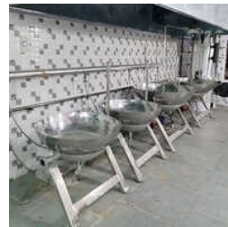
Wood Fired Steam Boiler Based Khoya
