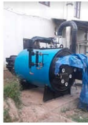
IBR Steam Boiler
