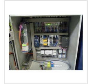
Industrial Control Cabinet
