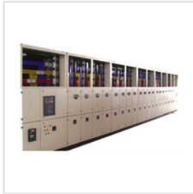
Industrial Control Panel
