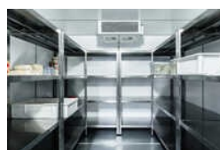
Frozen Food Cold Storage Room
