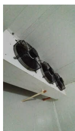
Cold Storage Rooms
