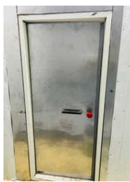
Ss Cold Storage Door
