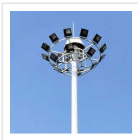
High Mast Street Lighting Poles
