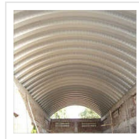
Self Supported Industrial Roofing
