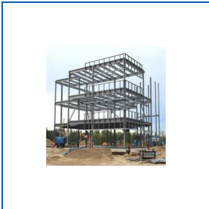
STEEL BUILDING FRAME
