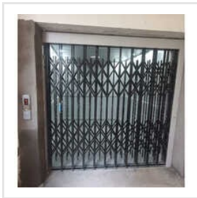
Industrial Goods Lift
