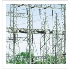
Hot Dip Galvanized Substation Steel
