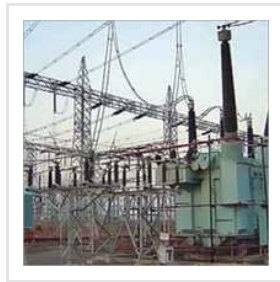
Power Substation Steel Structures
