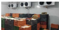
415V Cold Storage Room
