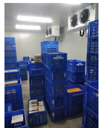
Mild Steel Cold Storage Room
