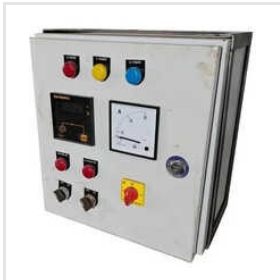
100A Electric Control Panel
