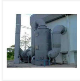
Industrial FRP Wet Scrubber
