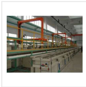
Anodizing Automatic Plant
