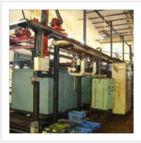
Hard Chrome Plating Plant
