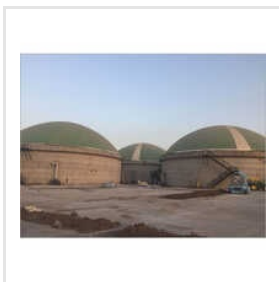
Bio CNG Gas Digester
