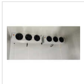
Industrial Blast Freezer
