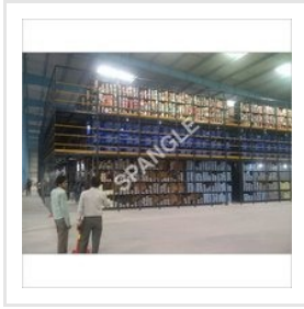
Three Tier Racking System
