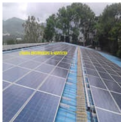
Industrial Solar Power Plant
