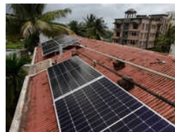
On Grid Solar Power Systems
