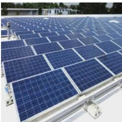
12v Solar Power System
