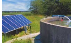
Solar Pump System
