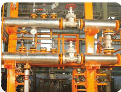
Skid Mounted Inlet / Outlet Piping System
