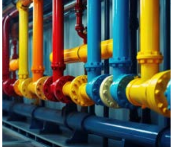
Hot pipelines & valves
