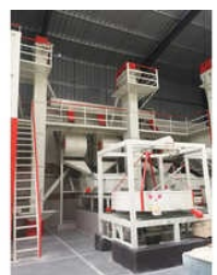
Industrial Peanut Shelling Plant
