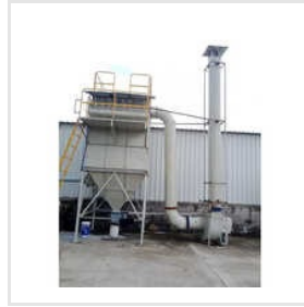
Dust Extraction Systems
