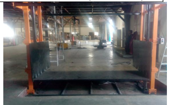
JI-175 Goods Lift (Double Mast)
