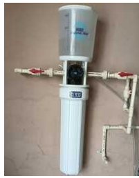
Domestic Water Softener
