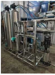
SS RO Plant
