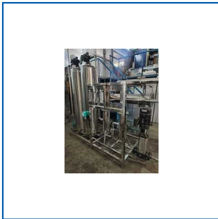
SS RO PLANT
